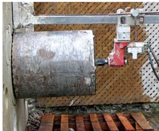
UT Engineering Students rigged electronic sensors to the anchor holding this 24-inch core drill rig mounted to a wall. The sensors measured the force that was put upon the anchor.
