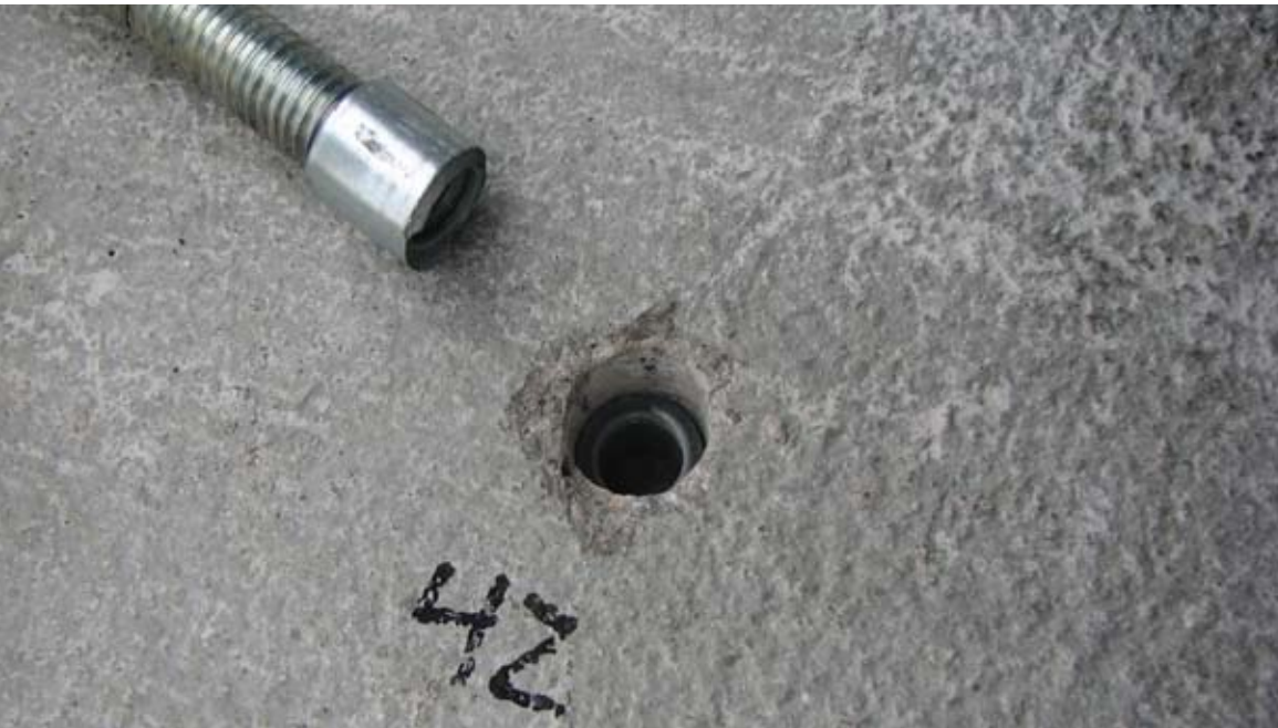
Anchor failures, such as these, were replicated by the students in field testing.
